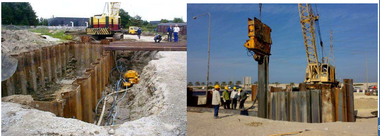
Sheet Piling Works For Water Pipe line Project @ Jubail With Yuksel Co.
