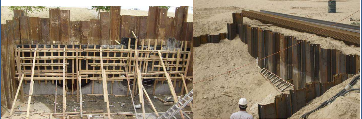
Sheet Piling works At (C-13) Pipe Line Work, Royal Commission-Jubail With Al Harbi Co.
