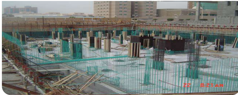
Shoring Works At Al Nimer Commercial Bldg, Near Movenpick Hotel- Al Khobar.
